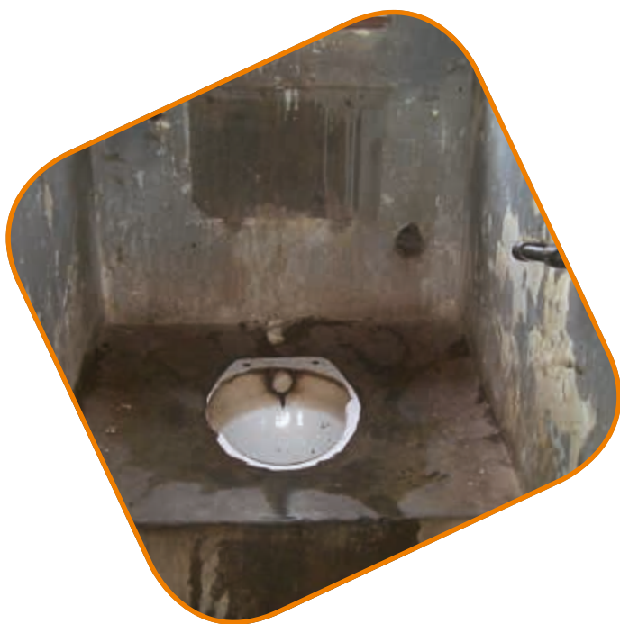
Photo: One of the two toilets used by 45 patients at Ndola closed male ward, 24 October 2012. © MDAC.
