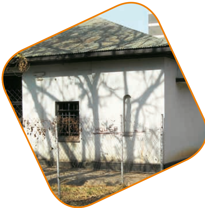
Photo: Ndola closed male ward with small prison-like windows and no outdoor space. The psychiatric facilities contrast with the main hospital visible behind, 24 October 2012. © MDAC.
